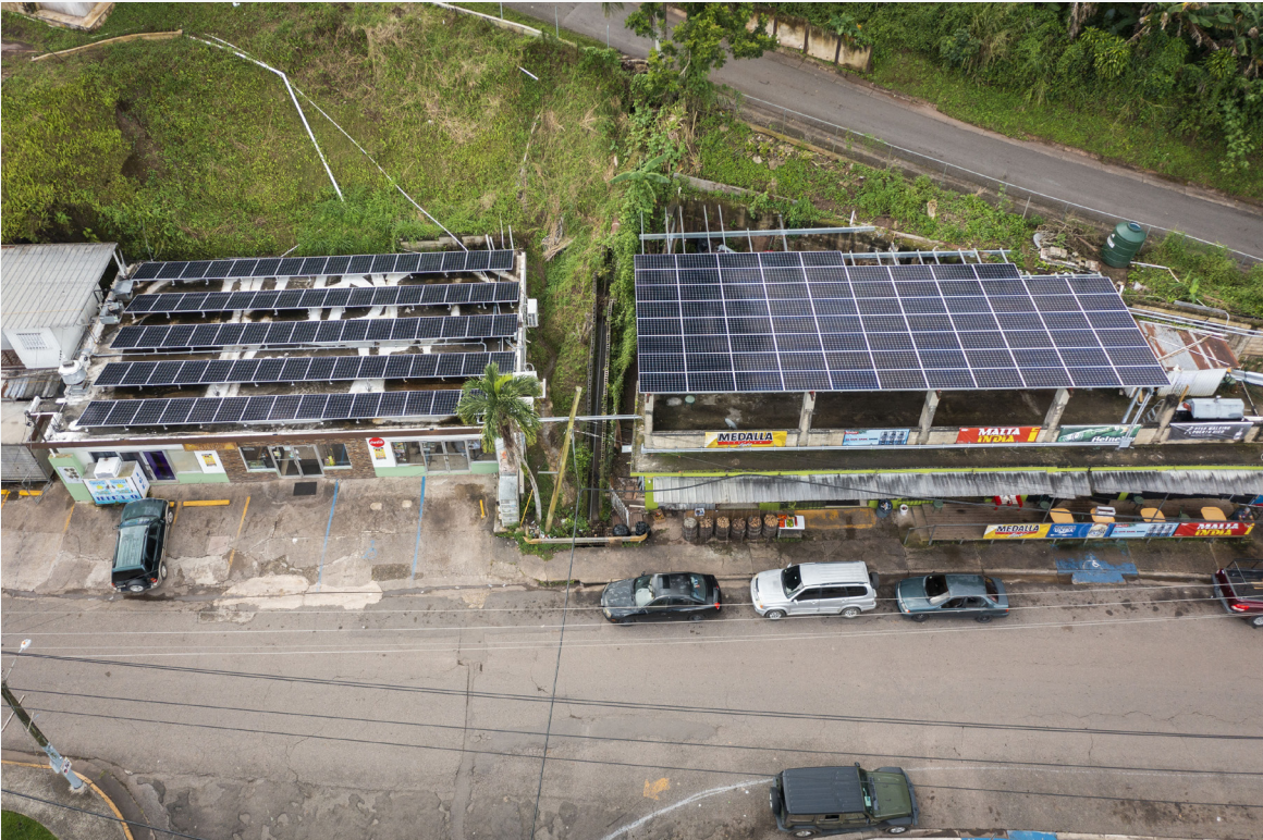
This microgrid system in Castañer, Puerto Rico, provided a rural community with backup power before, during, and in the aftermath of Hurricane Fiona in 2022. Alejandro Granadillo/Bloomberg via Getty Images
