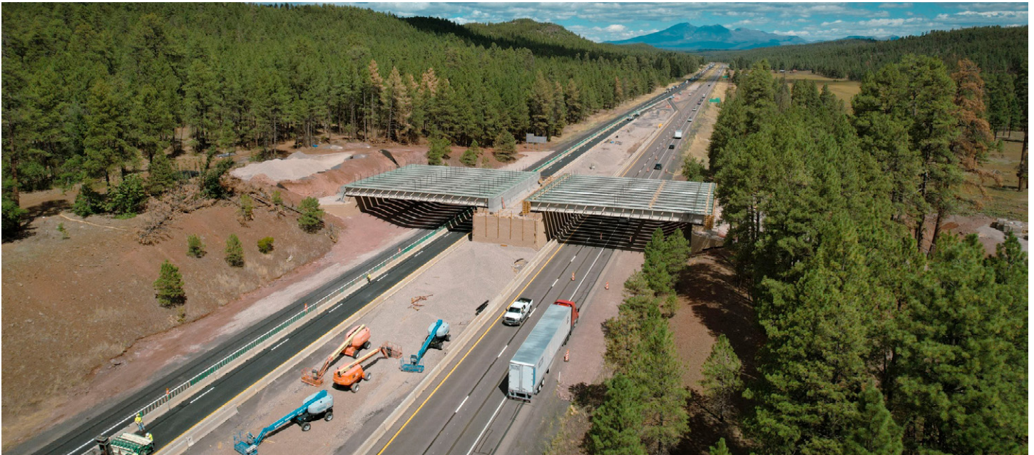
The Interstate 17 Willard Springs Wildlife Overpass, just south of Flagstaff, Arizona, will feature a 100-foot-wide vegetated bridge and 16 miles of fencing that also ties into existing culverts. Arizona Game and Fish Department
