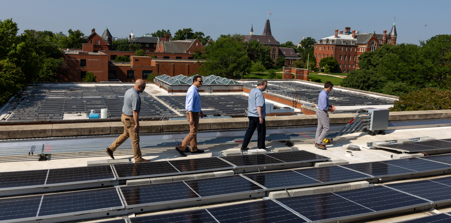
A solar array atop a Gallaudet University building generates clean energy that feeds into the local grid and helps provide electricity for residents and neighboring businesses. It also provides power for much of the campus; in an outage, energy stored in batteries could provide electricity for the whole college. The Pew Charitable Trusts
