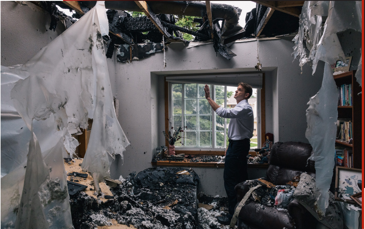
Battalion Chief Erich Roden looks over the fire damage to a townhome after lightning struck an external gas meter in the early hours of the morning during a storm.
